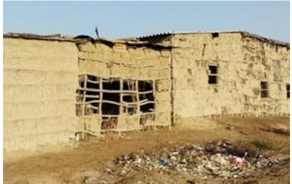
Fig 55 Shop owner removed mud plaster to capture wind inside shop. Source: Captured by Author
